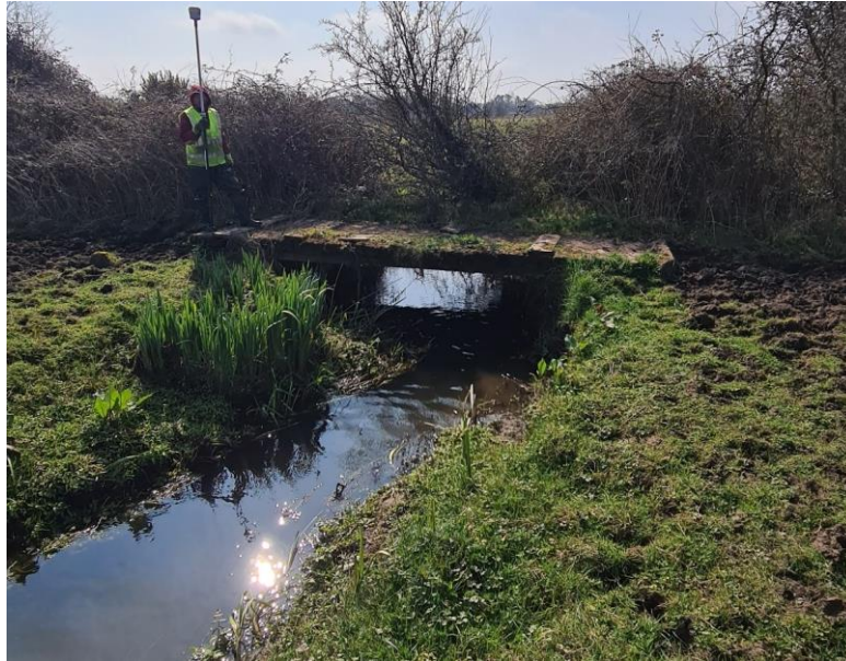
Figure 2.1. Bridge 17-Farm Access road concrete bridge single span c. 4m wide (u/s elevation)
